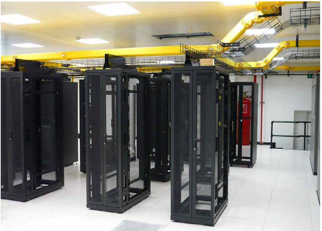
Typical installation of overhead copper and fibre management system with customised brackets to the top of the cabinets
